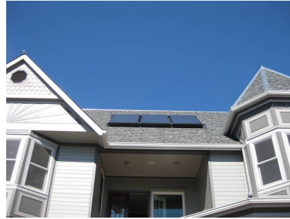
SE Facing Roof (Flat Plate)
