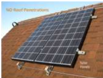
TCS Roof Mount with a 270 Watt solar array
