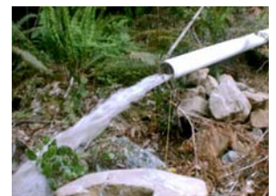
First Flow at the powerhouse site of the OP's latest hydroelectric system
